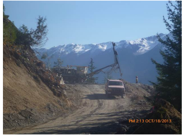
Photo 2. Drilling activities at the west heading of the Truckwash Creek FSR realignment (Oct 18, 2013).
