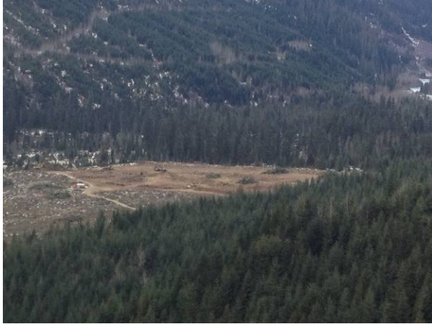
Photo 3. Overview of grubbing activities completed at the future construction camp location (Dec 10, 2013).
