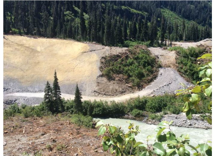
Photo 4. Construction underway for temporary haul road. Hydro-seeding has not successfully germinated at the ULRHEF intake diversion (July 9, 2014).
