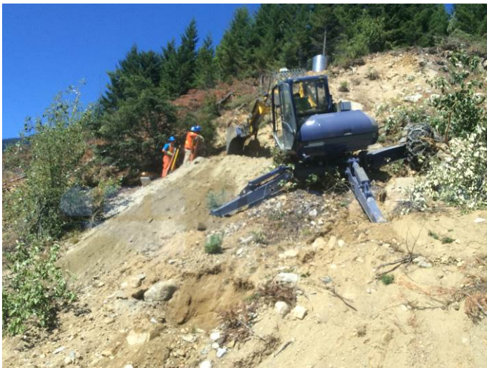
Photo 5. Pole foundation installation in Segment 2 with an excavator capable of working on steep slopes (July 9, 2014).
