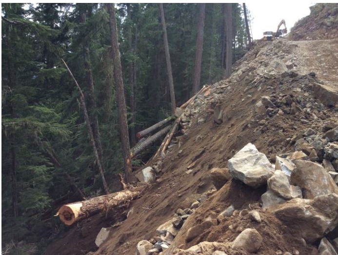
Photo 1. Boulder Intake Access road construction practices that did not conform to the work plan and resulted in a Stop Work Order by the Owner and IE. (July 21, 2014).
