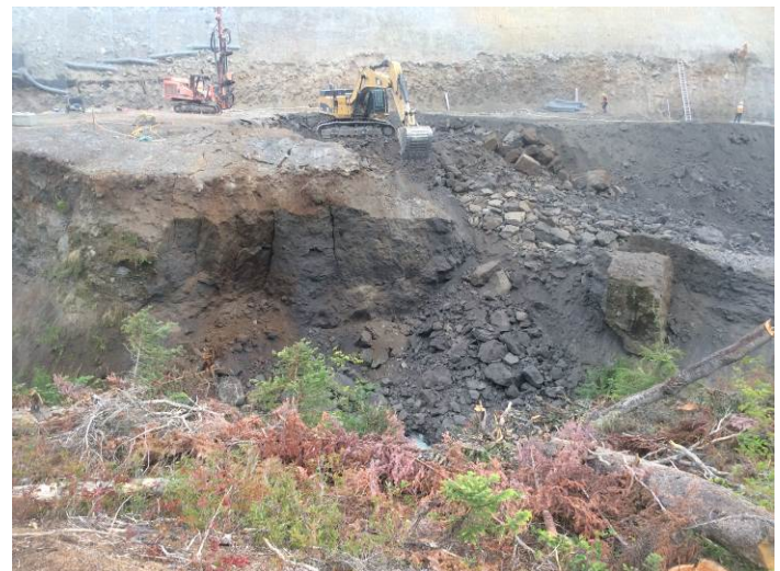
Photo 4. Excavation of blasted rock at the ULR intake diversion channel. Minor amounts of rock fell into the Lillooet River during monitoring of the works. (July 23, 2014).
