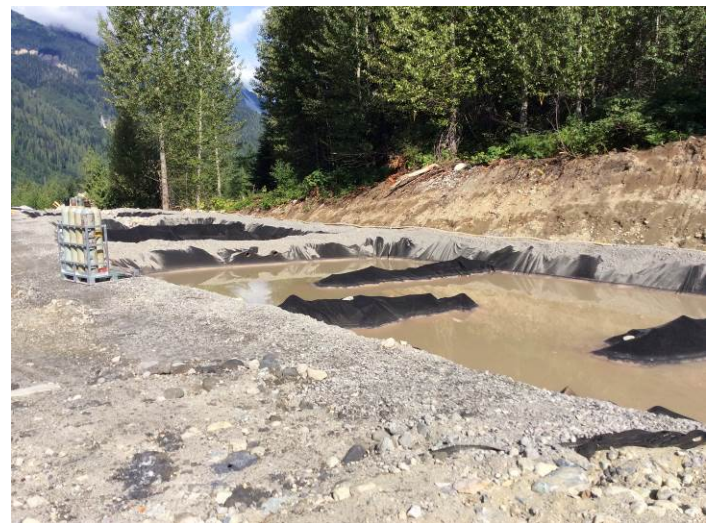
Photo 2. Dewatering of seepage from the tunneling activities was performed this week but the water has not yet reached the second treatment pond (July 19, 2014).
