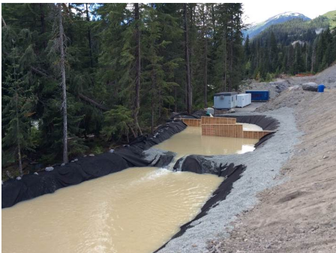
Photo 3. Sediment ponds constructed to for the treatment of dewatering the ULRHEF powerhouse excavation (July 25, 2014).
