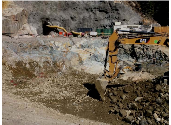
Photo 2. Dewatering of seepage from within the powerhouse excavation was pumped to the sediment ponds. Water has not yet reached the second treatment pond (August 9, 2014).
